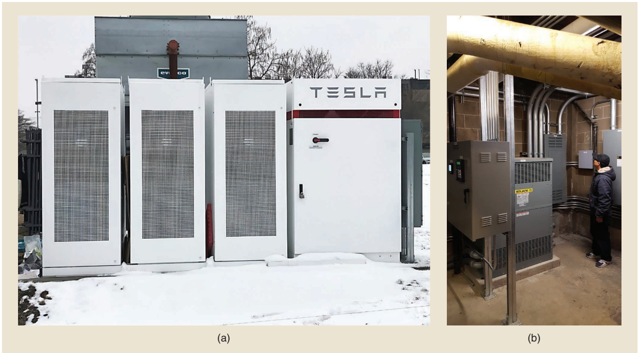
Figure 7. The (a) battery storage and (b) power electronics control room.
