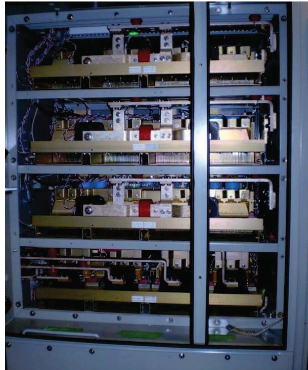
Figure 11. The ±1.25-MVA SMS inverter and two choppers. (Image courtesy of S&C Electric, “Storage Management System,” http://sandc.com/products/energy-storage/sms.asp .)
